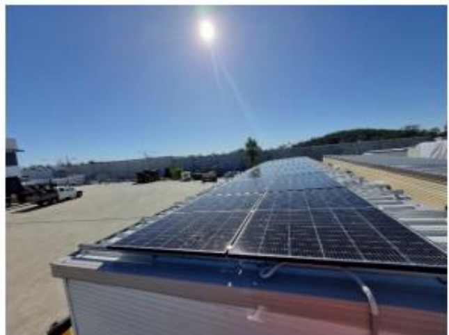
Figure 4: Solar Cells on accommodation dongas.
